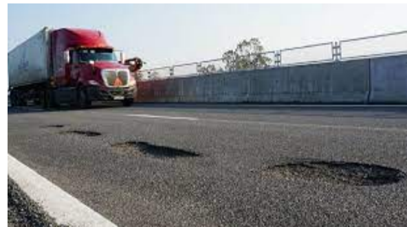
Figure 1. Crack and potholes were seen at Da Nang - Quang Ngai expressway [13].
